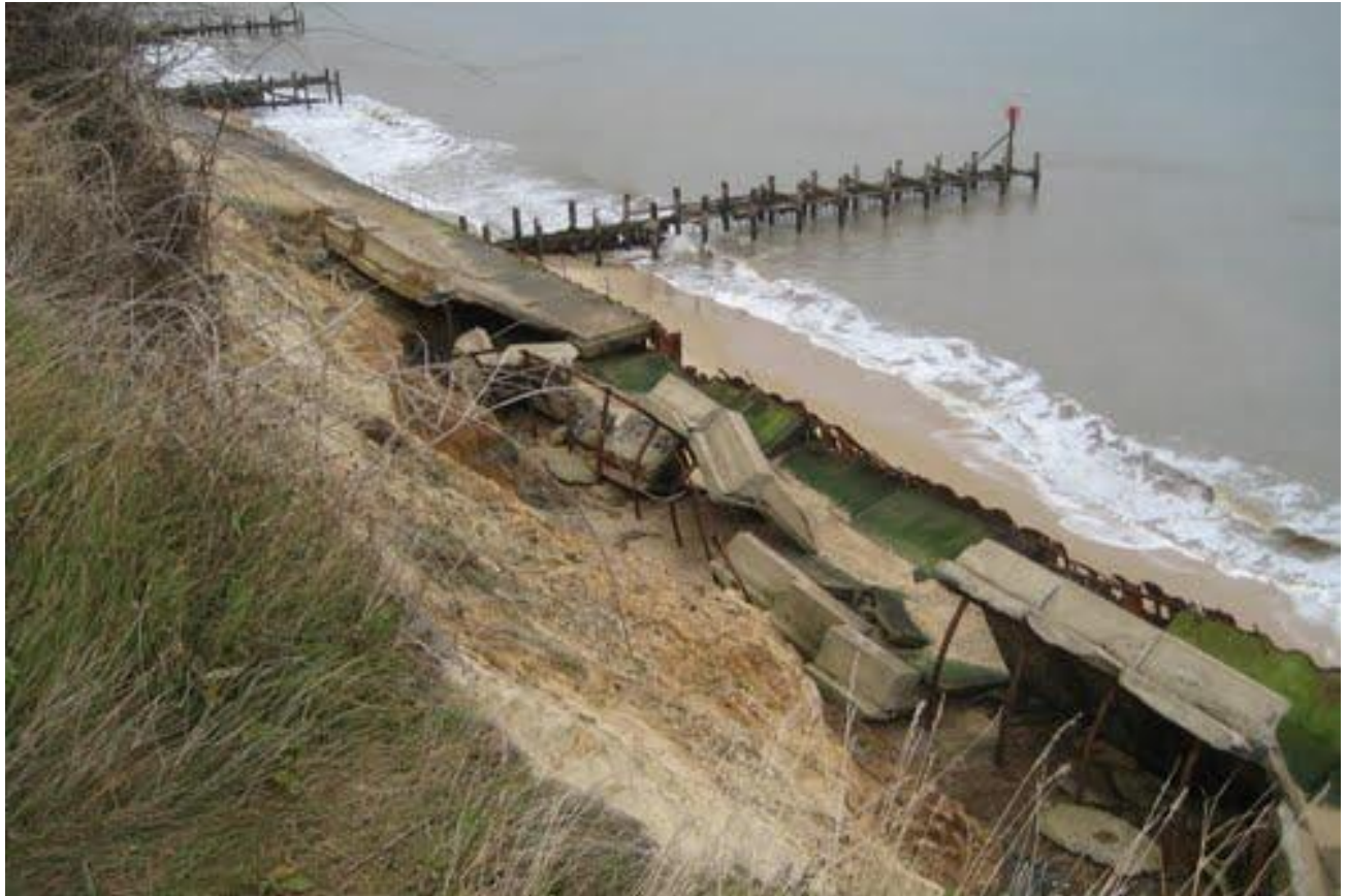
Figure 50. Site 9. Google Earth Panoramio photograph showing damaged sea wall near Site 9. There is now no pedestrian access either along the cliff top or down on the beach except at very low tides with difficulty.
