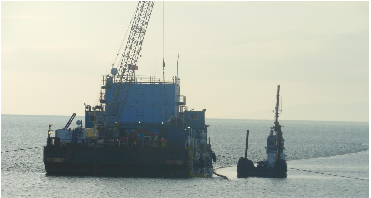
Figure 20. Large barge with four point anchoring and workboat. On the right hand side of the barge the duct can be seen being pulled into the HDD. The water depth is approximately 4m.
