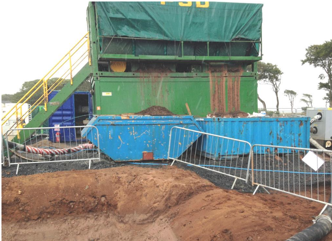
Figure 15. A drilling fluid recycling unit with hydrocyclones and shaker screens on the upper level and active mud tank underneath. The blue bins capture cuttings as they are removed by the shaker screens. On the right is a grey transfer pump for transferring cuttings from the entry pit (foreground) to the hydrocyclones and shaker screens.
