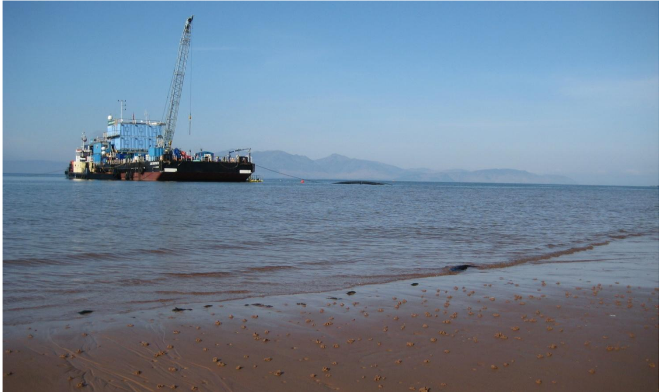
Figure 11. Barge in position during installation of ducts for the Western Link HDD Landfalls.
