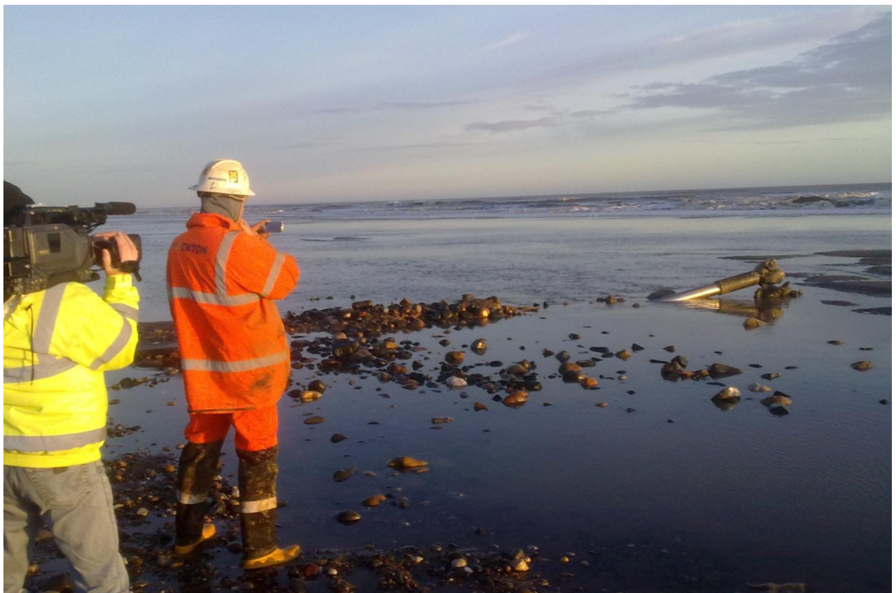
Figure 10. HDD exit on the Humber Gateway project illustrating the short HDD option of exit near MLW.
