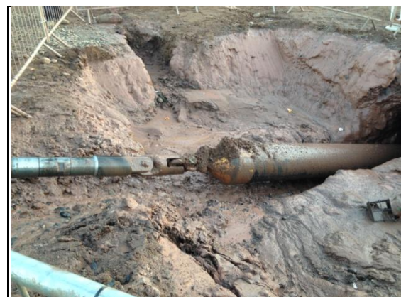
Figure 19. Drilling rod, swivel, pulling head and duct being pulled into the entry pit
