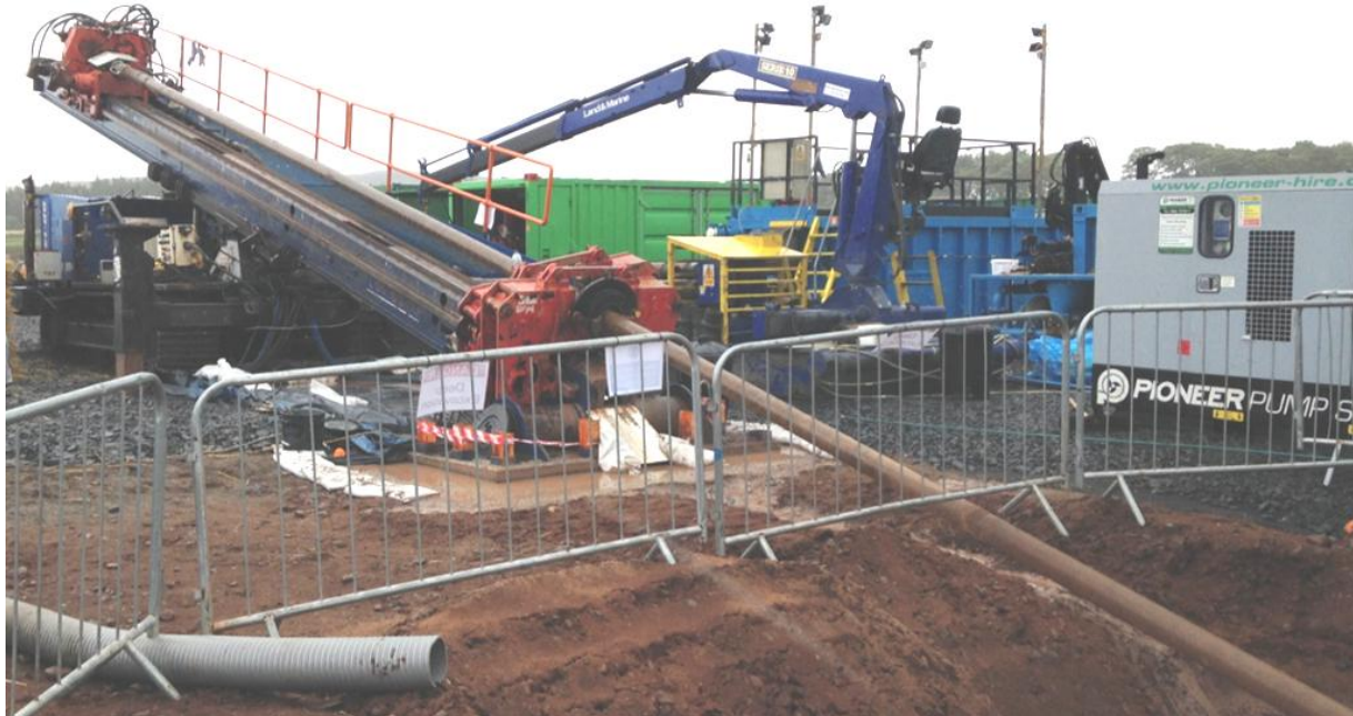
Figure 13. Example HDD rig of similar size to that required for the HDD's.
